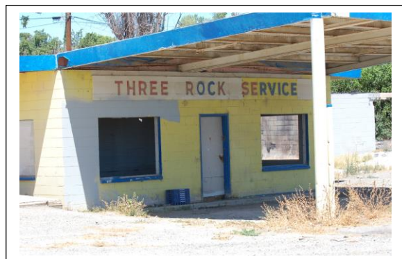
Abandoned service station on W. Panoche Road in western Fresno County. The service station had sunk partly into the ground as a result of land subsidence due to over-pumping of groundwater.
