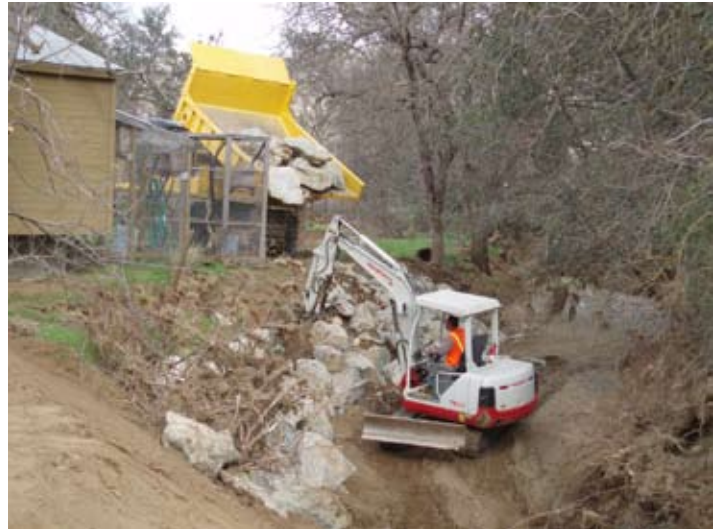
A front-end loader carefully places large, angular rock along the creek bank beneath Stallings' home. The equipment rides on rubber tracks that put only 8 psi of pressure on the ground, reducing soil compaction.
