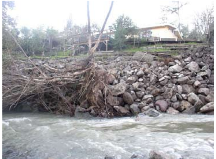
The creekbank protection project, as installed. The work was completed by January 21, 2006.
