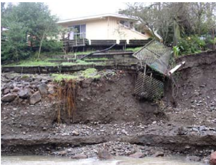
Damage due to the flooding of Sonoma Creek endangered the home of Glen Ellen residents.
